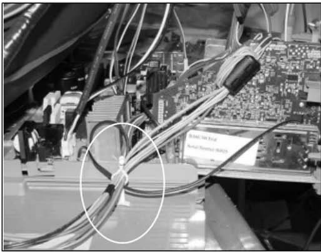
Dress HM board grounding wires, A board lightning wire, 12P video harness (M~HU board) and 12P (HM~M) together into standing purse lock.
